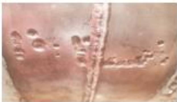
Fig. 4. Pipe corroded before corrosion protection
