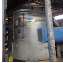
Figure 7. Tank Pellet Dryer
