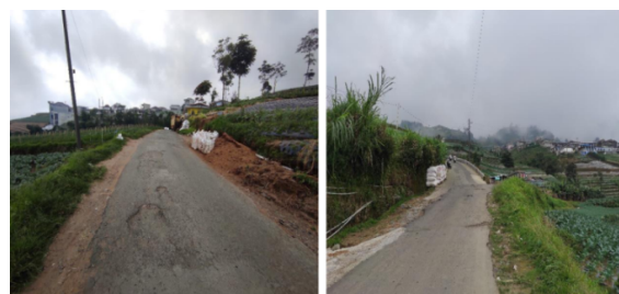
Figure 1. Condition of Access Road to Nepal Van Java
