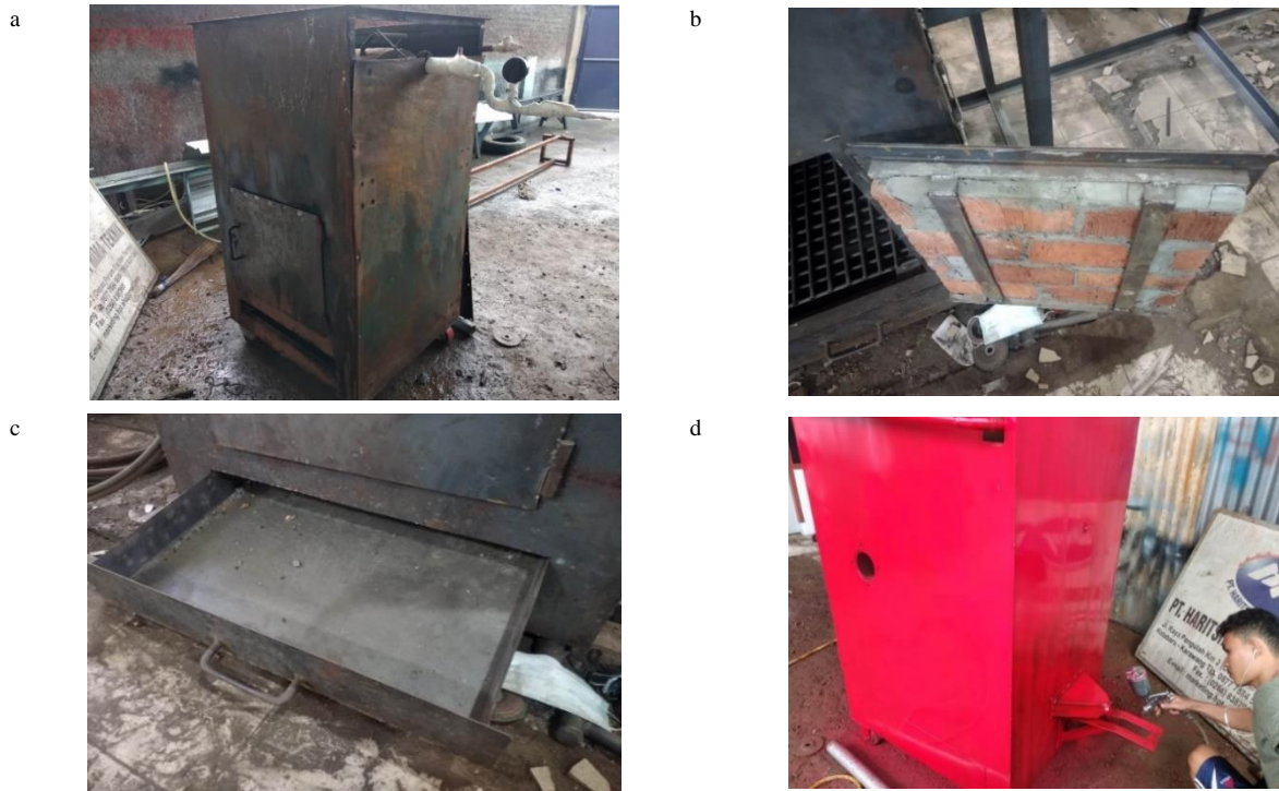
Figure 3. (a) Incinerator casing; (b) Incinerator door; (c) Ash storage; (d) Painting process
