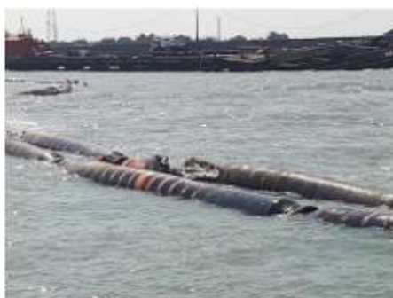
Figure 1. Floating Hose damaged due to tangling (PT. KPI Unit VI Balongan)
