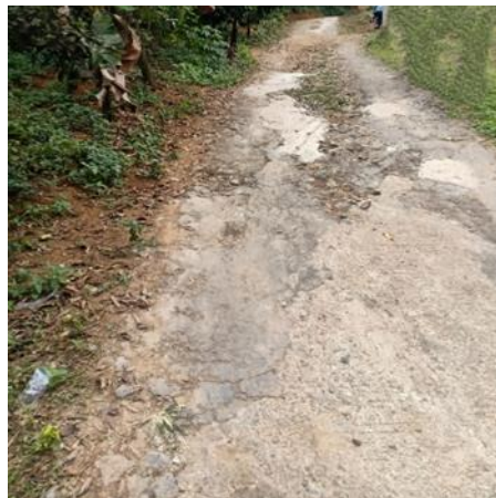
Figure 1. Road condition at Kp. Jukut Pandeglang
