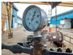
Figure 4. The Pressure rate at Holding Time for more than 1 hour
