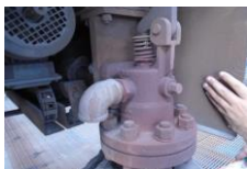
Figure 14. The Physical condition of vent valve on one of PS-SL sootblowers
