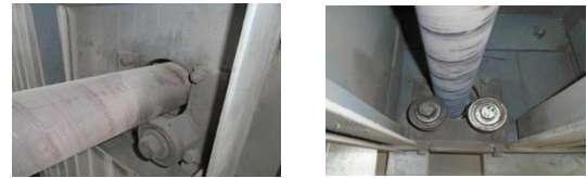
Figure 3. Lance tube sootblower PS-SB that is not centered
