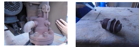
Figure 4. The physical appearance of the vent valve on one of the PS-SL sootblowers
