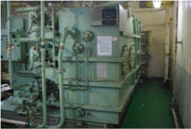
Figure 4. Bulging on Sewage Tank
