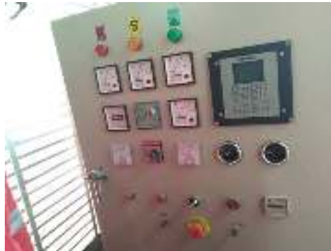
Gambar 6. Panel Pengontrol Genset
