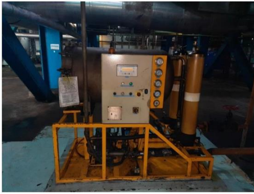
Figure 8. Purifier MOT Unit 3
