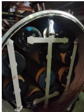
Figure 14. Inside of the Coalescent Filter
