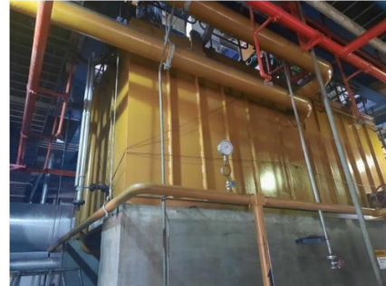
Figure 2. Main Oil Tank
