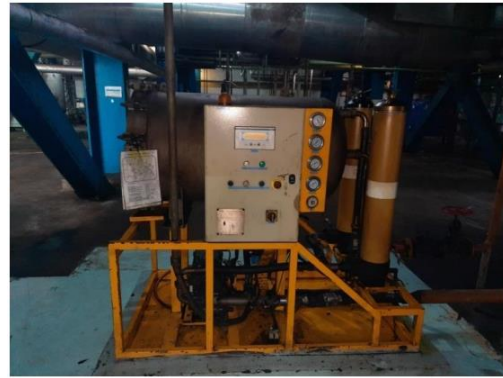
Figure 7. Oil Purifier System
