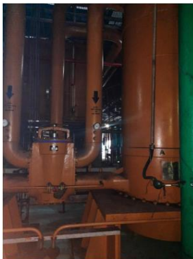
Figure 6. Lube Oil Cooler
