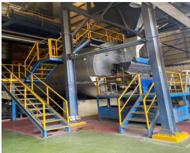
Figure 2. Fire Boiler Tube PT.Sinar Meadow
