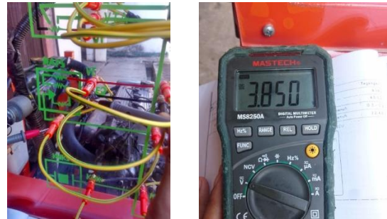
Figure 6. Checking the PIM-E2 terminal voltage
