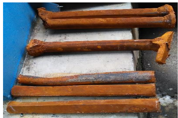
Figure 9. Damage to the Support Coupling Bolt
