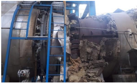
Figure 5. Damaged Cover Insulation
